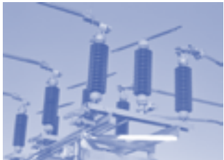
High voltage isolator © Econnect Ltd
