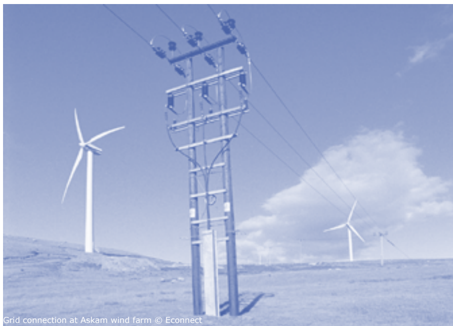
Grid connection at Askam wind farm © Econnect
