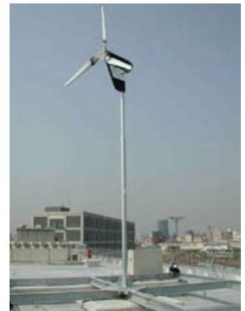
City rooftop installation © Prove Energy
